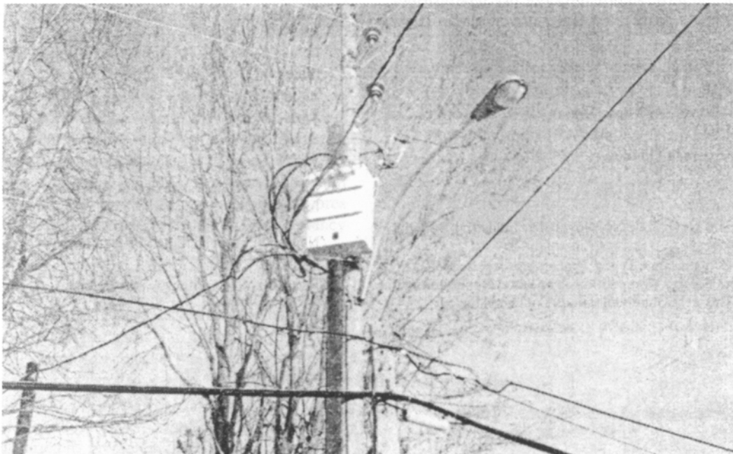
Fig. 3 Pole-type amorphous-core distribution transformer on Hydro-Québec power system
